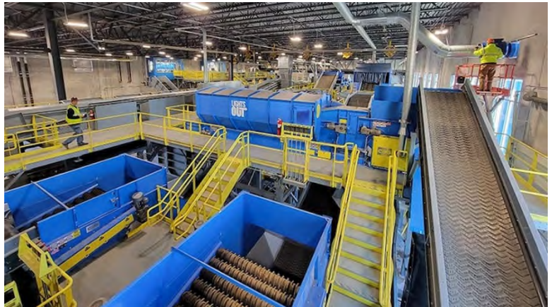
Figure 3.9 Typical MRF Facility (Courtesy CP)
